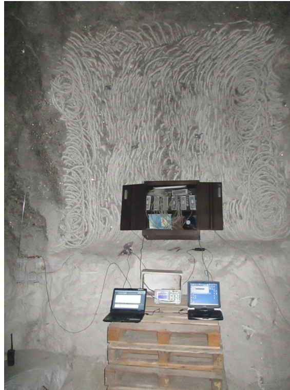
Fig. 3. The monitoring station equipped with the AE piezoelectric sensors, the telescopic antenna and oscilloscope for EME evaluation, and the NE proportional counter.
